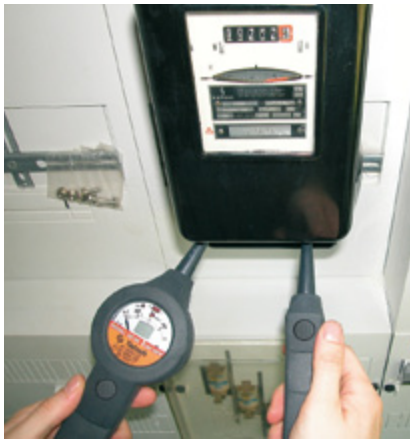
Integrated 350W-load for fast start-up tests at electricity meters
