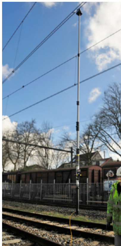
Test at a rail overhead line
