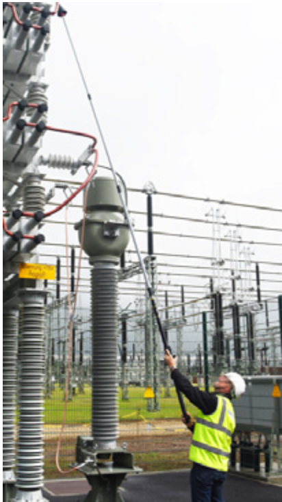
Test at a 36 kV compensation system
