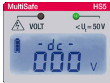
Indication of absence of voltage
