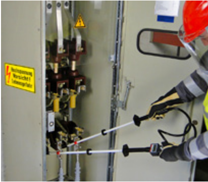
Test with HS 11 at 10 kV transformer
